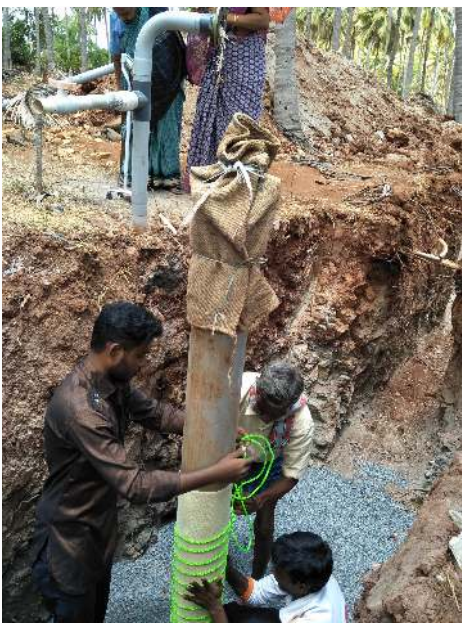
The bore well recharge process
