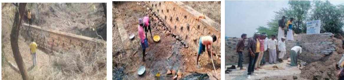
Peta-Alur and Harogeri Check dams handed over to the villagers on World Water Day.
